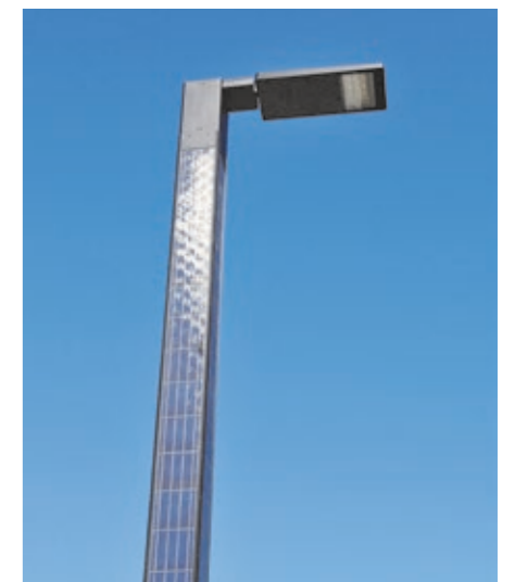
Street lamp with solar.
